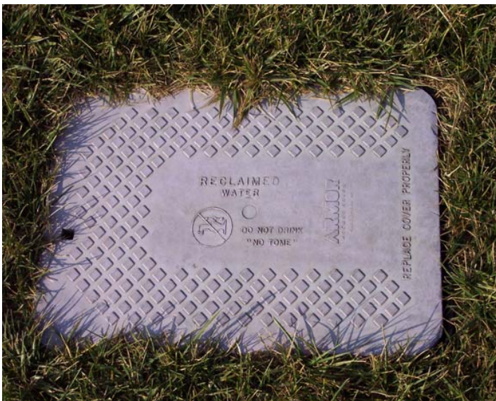
Valve boxes noting the use of reclaimed water
